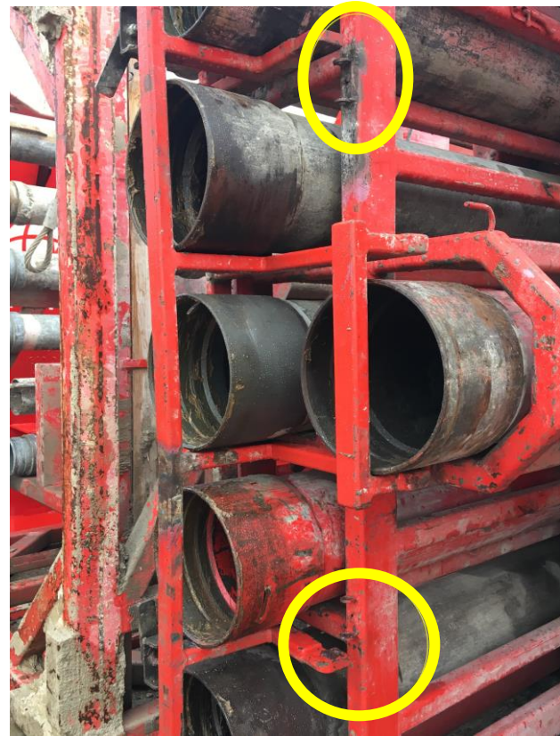
Tremie rack involved in the incident
