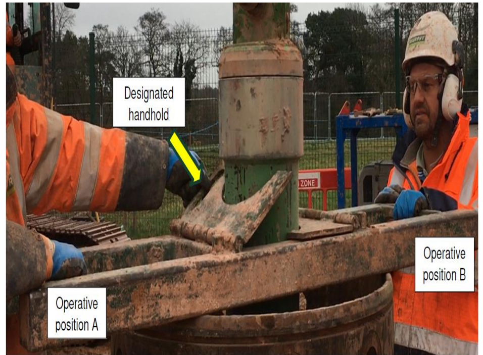
Tremie pipe being lowered to the suspension jig above pile casing / Correct positioning of operatives
